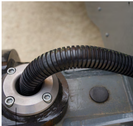
Excellent protection for exposed cables
